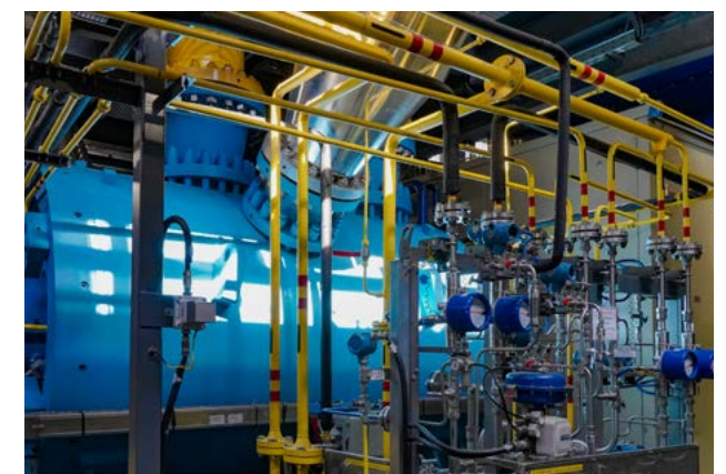
Mixed refrigerant centrifugal compressor K 905-71-1C at Cryogaz Vysotsk LNG PLant
