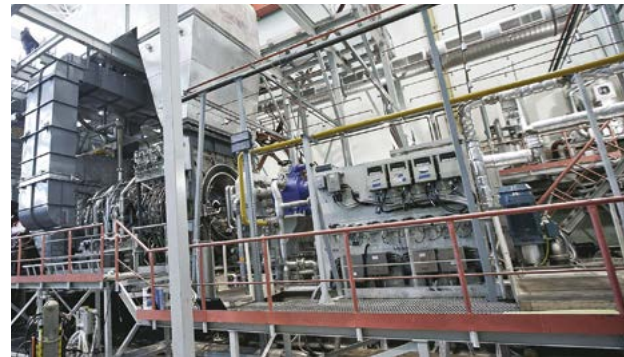
32 MW gas turbine test bed
