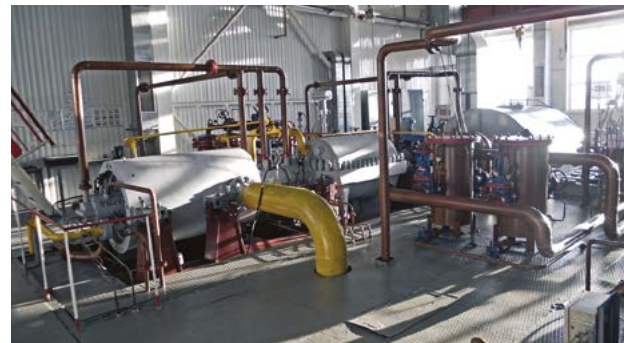
Centrifugal compressor K320-131-1 at CS of Severo-Danilovskoye Field TPE
