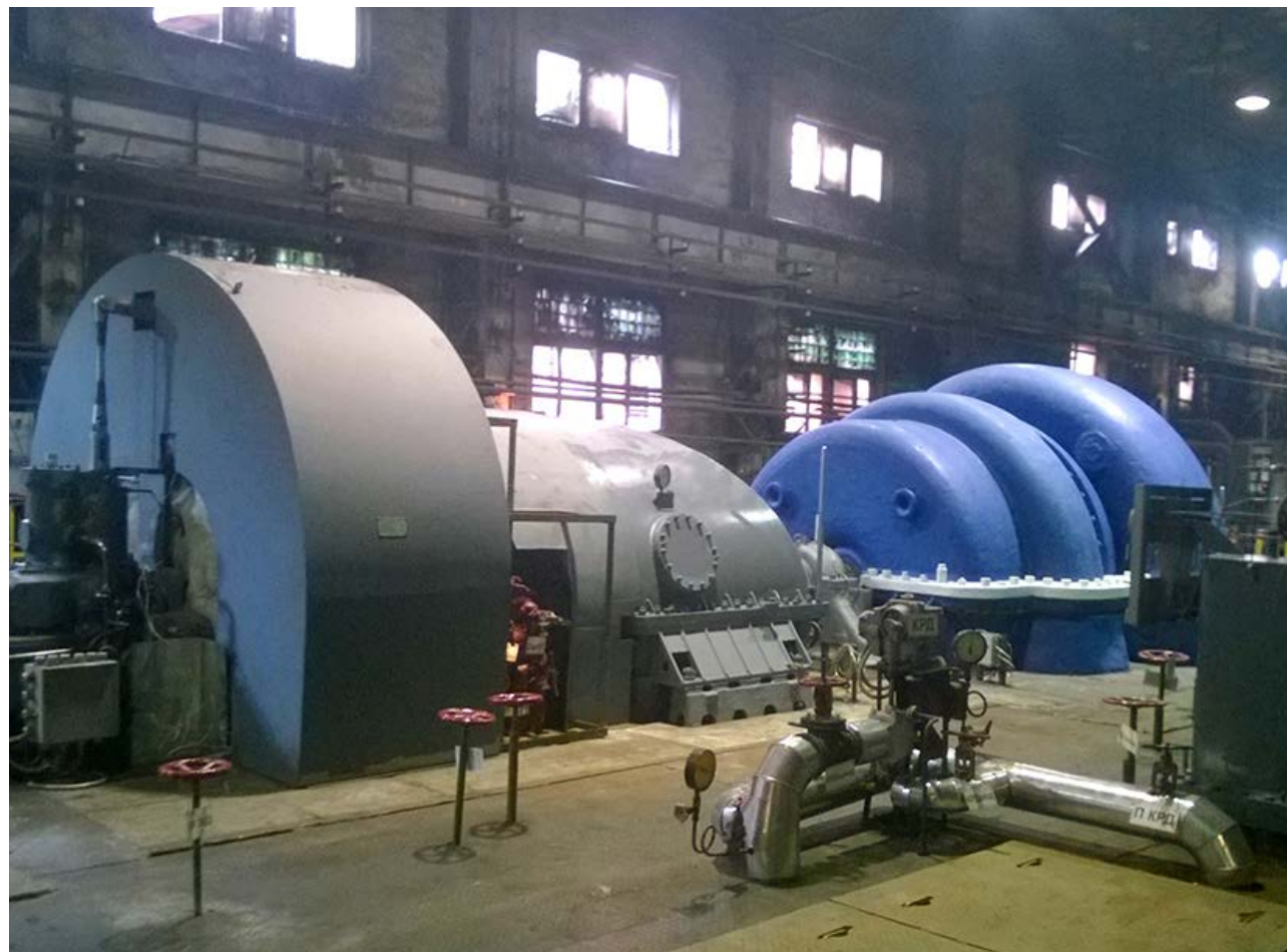
5200/25 Turbocompressor Unit with automatic control and monitoring system at Magnitogorsk Iron and Steel Works
